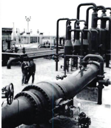
A natural gas pumping station in Sichuan Province. Sichuan currently produces about half of China's gas and hopes to import modern technology to help it double output by the end of the decade.
