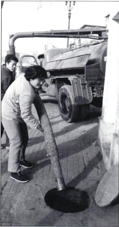
Sanitation engineering is primitive in China, as evidenced by these workers cleaning city sewers in Jinan, Shandong Province.
