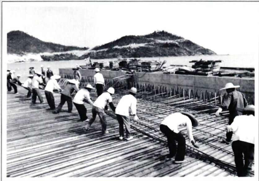
Work is proceeding rapidly on the deep-water berth for 10,000 dwt vessels at Chiwan, where the South Sea Branch of the China National Offshore Oil Corporation plans to build a major supply base.
