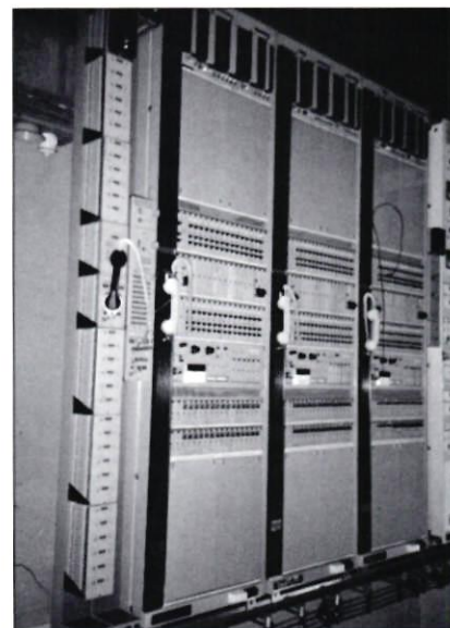
Optical fiber waveguide terminal 480-channel equipment bay in Wuhan.
