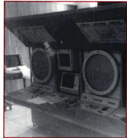
The area control center houses five long-range secondary surveillance radar consoles, two of which are in operation.
